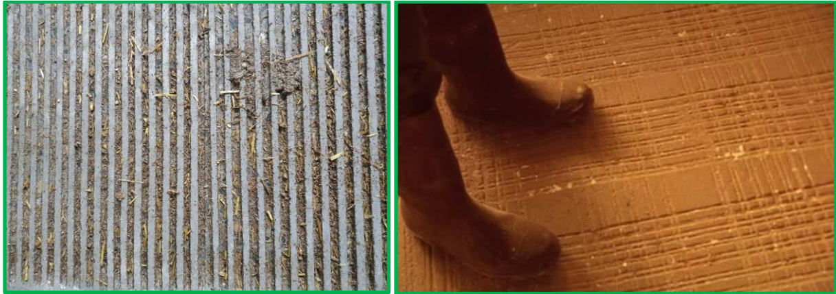
Good non-slip flooring (concrete with slots milled out) at Feenstra slaughterhouse (left) and unknown slaughterhouse (right)
