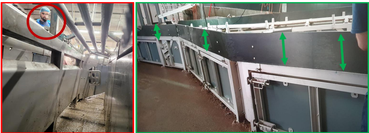
To prevent pigs from seeing workers ahead (left photo), Compaxo slaughterhouse in Zevenaar (NL) placed “wooden view shields” all along the entire length of the single-file raceway (right photo). When workers stand behind these shields, the pigs in the single-file cannot see them as easily.
