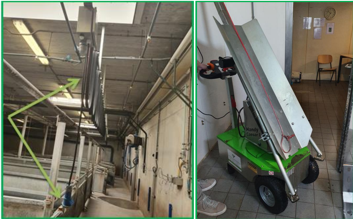
Left: cord and socket attached to a rail along the entire lairage so the mobile electric stunner can be used everywhere in the lairage. Right: mobile trolley to bring pigs that have been emergency stunned and bled-out pigs to the slaughterline.
