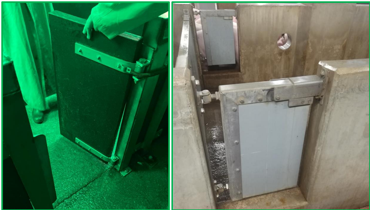
Doors in the lairage pens so aggressive or attacked pigs can be removed easily
