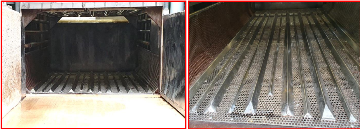
When there is a sudden change of flooring (from concrete to shiny metal) pigs will balk. Especially at high speeds, this can cause serious problems. Additionally, the cleats are also placed in the wrong direction, which results in suboptimal grip.
