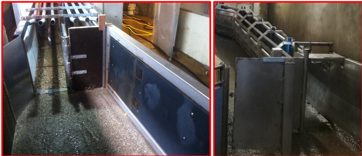
Raceways with a “cage-like tunnel construction” do not work as well as raceways with an open top. They cause shadows on the floor and gives pigs the feeling of being trapped.
