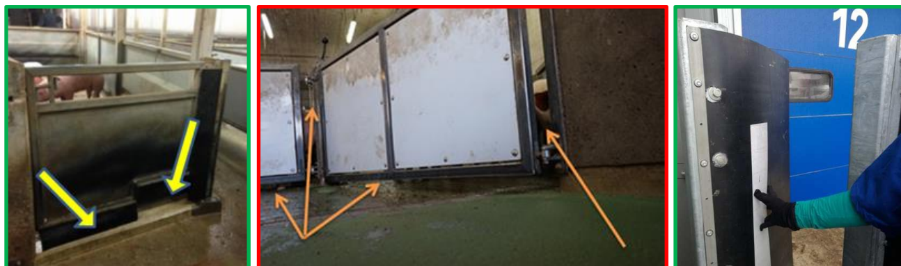
Good anti-draft rubber curtains at Westfort pig slaughterhouse in the Netherlands to stop drafts (left photo), open gaps causing unwanted drafts (middle photo) and a curtain (right photo) to block distractions and unwanted drafts into the lairage.
