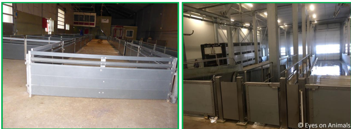
Plastic gates are much better than metal one to keep noise level low: at export center Meijer (left photo) and slaughterhouse Westfort (right).
